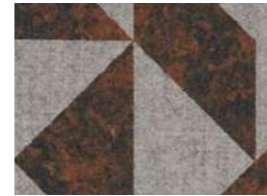
Corrosion View Options
